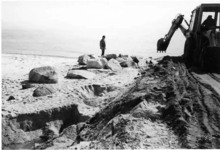
Bike path repair near Trunk River. Photo by Donald J. Zinn, courtesy Margery Zinn.
