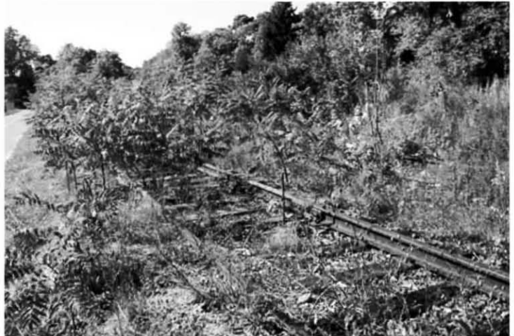
Rail at siding near former Grain Mill shows through weeds alongside bike path extension. Photo by Janet Chalmers.
